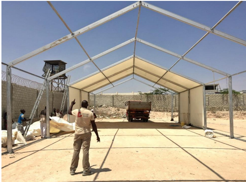
A Mobile Storage Unit is erected in support of the humanitarian community in Somalia.
